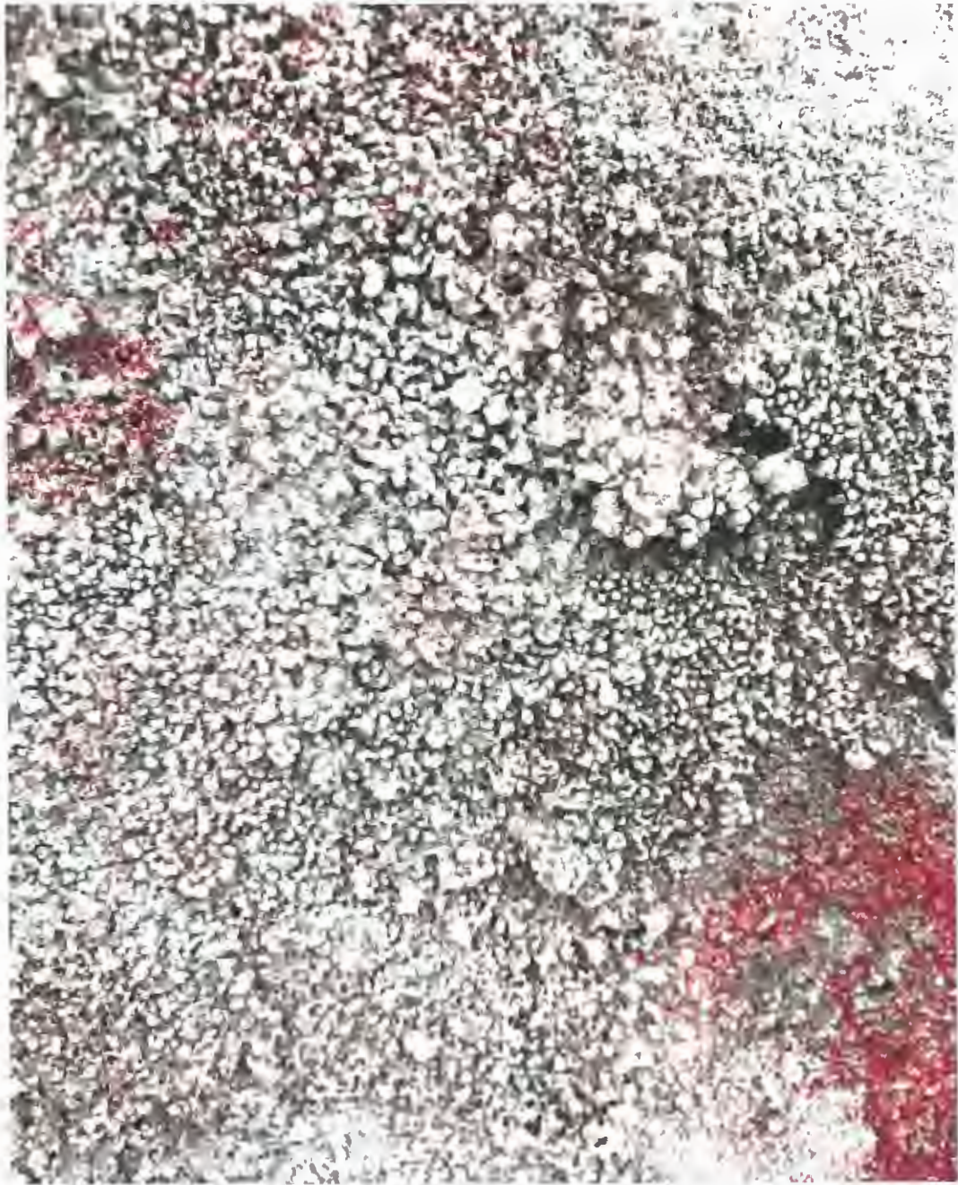
Figure 11. Detail of multiple layers of crystallized salt on surface, 2017
