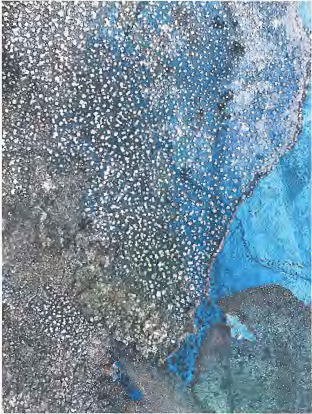
Figure 12. Detail of crystallized salt on surface, 2017
